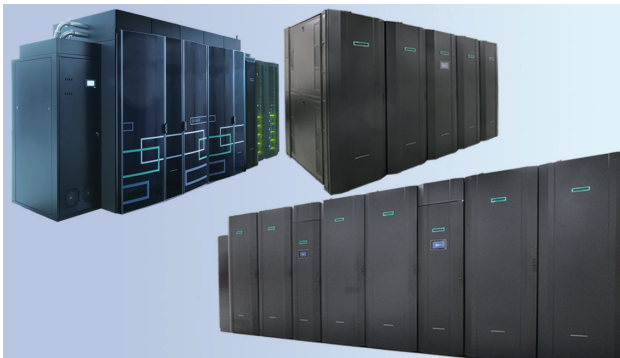
Supercomputer System for Statistical Science (top left), Communal Cloud Computing System (top right) and Supercomputer System for Data Assimilation (bottom right)
